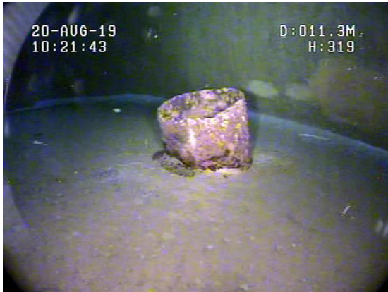
Inlet-outlet pipe appears corroded
