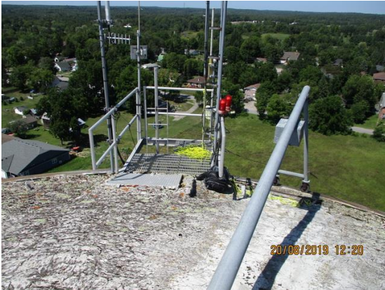
View top side landing and hoisting structure
