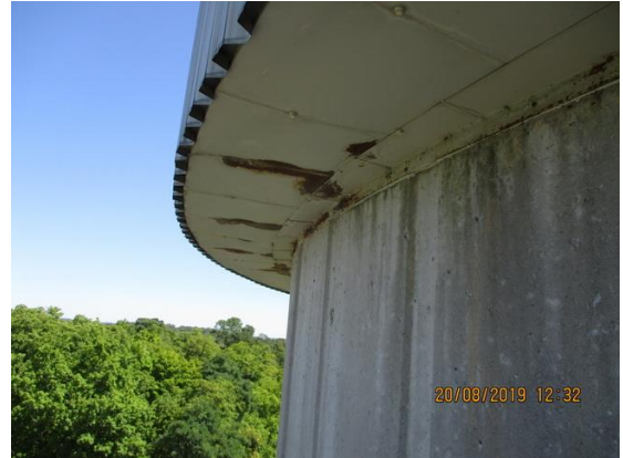
Sheet metal joints stained under tank edge
