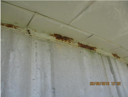
Underside of tank edge insulation sheet metal corroded
