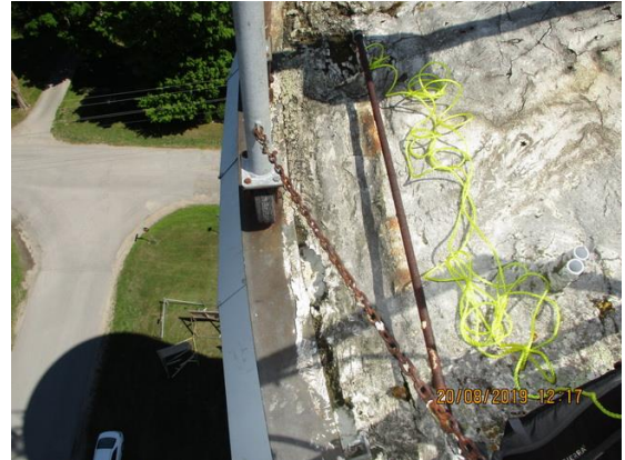
Tank roof edge near ladder; some insulation damage
