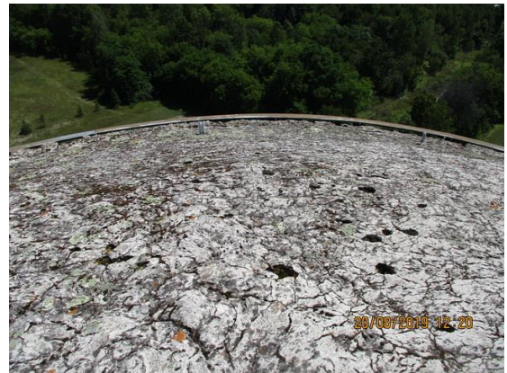
Tank roof section; some areas of insulation damage
