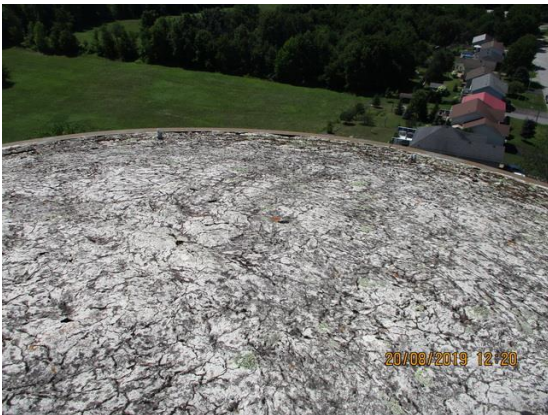
Section of tank roof topside insulation
