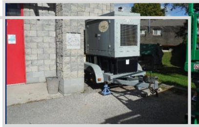
Automatic Back-Up Generator
